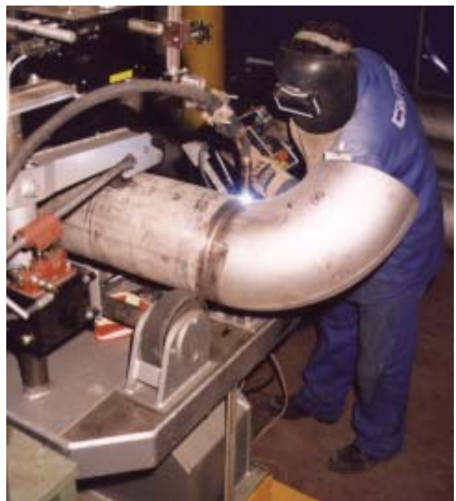
Figure 2. A complete ESAB solution for the mechanised TIG welding of stainless pipes.
