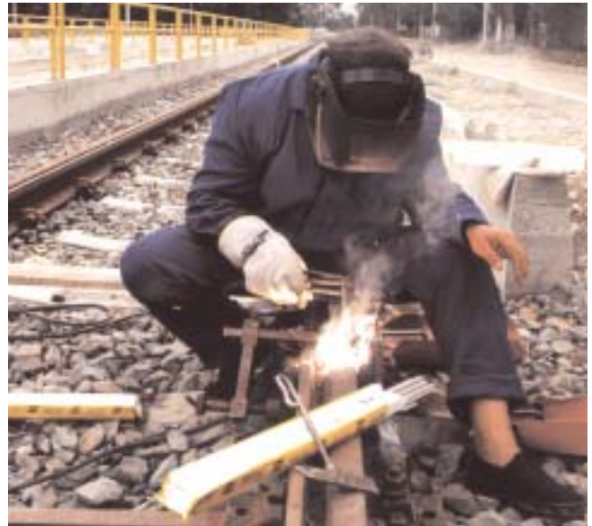
Figure 5. Mould welding with OK 74.78. Note the use of electrodes from VacPac vacuum packaging.
